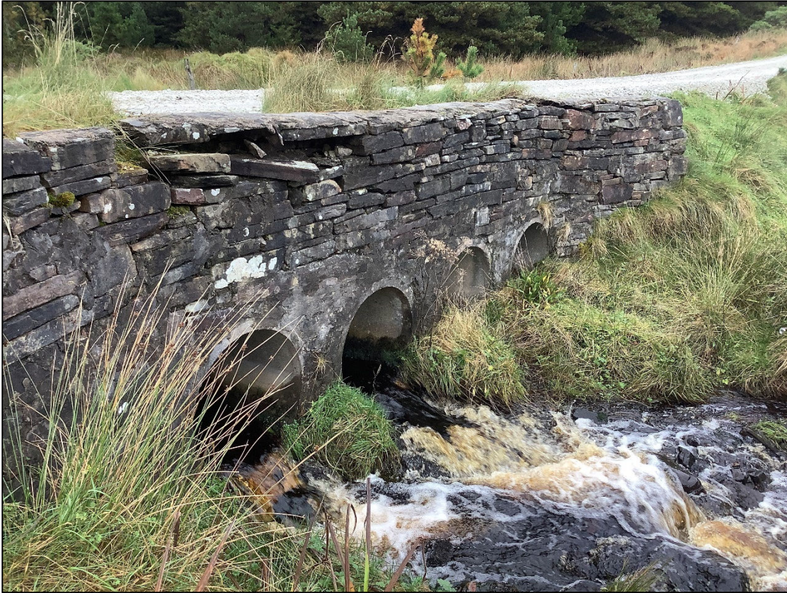
Plate 13-47: Northern end of grid connection route located at bridge 122m south of proposed substation location.
